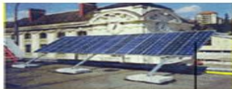
Generasi ke 1 Panel PV mounted
